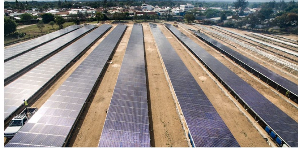
▶ A solar farm will partially power our South African data center campus.
