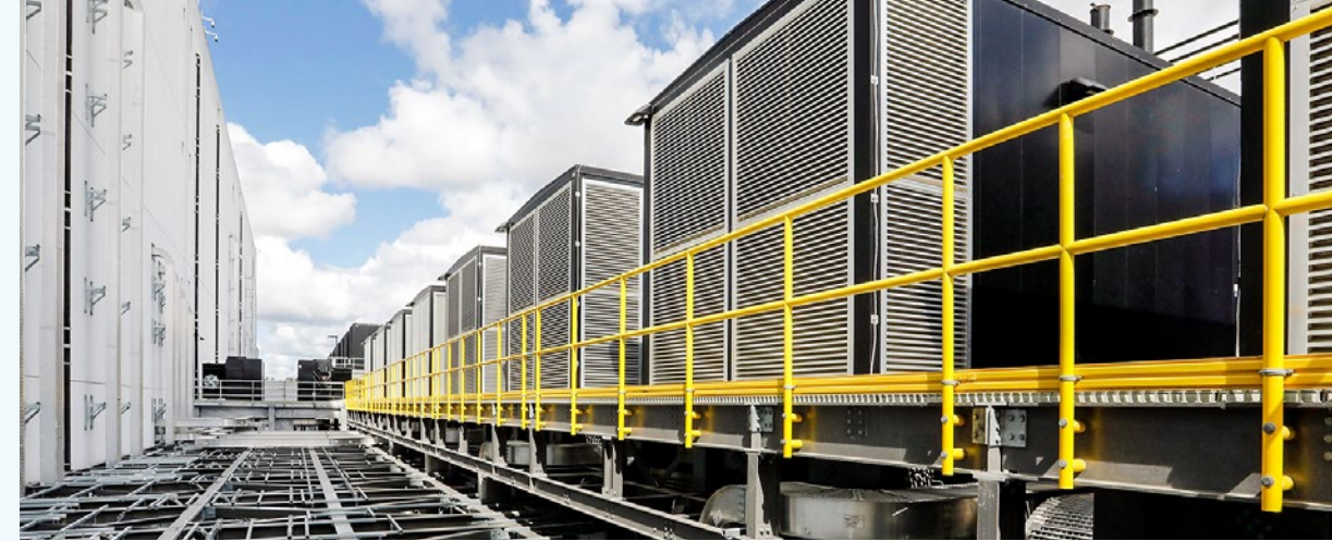
► FRP supports at our Santa Clara II campus.
